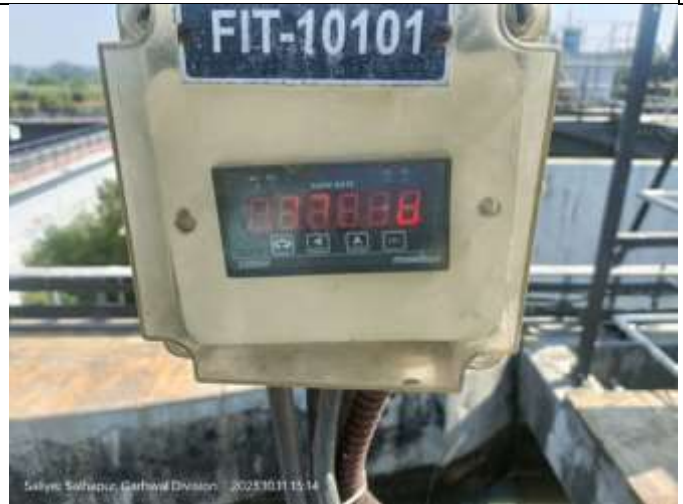
Fig 2: Inlet flow meter
