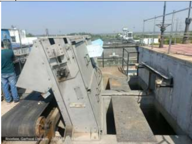
Fig 1: STP inlet screen
