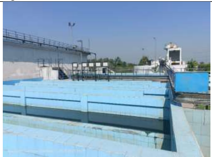
Fig 4: Chlorine contact tank
